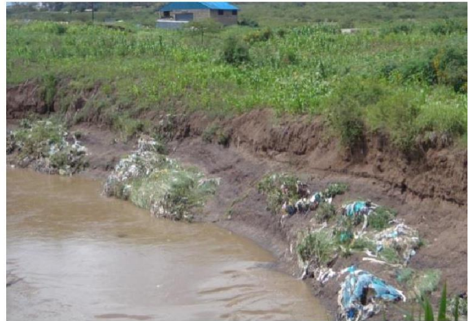
Figure 10. Basal Cleanout of the outer bank. Monene, 2014: Photographs were taken near Kangundo Road Bridge on 28/12/2012.
