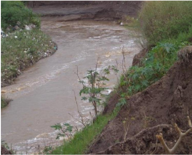
Figure 11. Undercutting of outer bank. Source: Monene 2014: Photos taken on 17/12/2013 during wet season) and 5/9/2013 during dry season.
