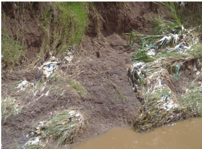
Figure 9. Basal Cleanout of the inner bank. Monene, 2014: Photographs were taken near Kangundo Road Bridge on 28/12/2012.
