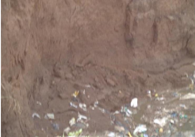
Figure 8. Collapsed outer bank. Monene, 2014: Photographs were taken 10 m downstream of Kangundo Road Bridge on 17/12/2013.
