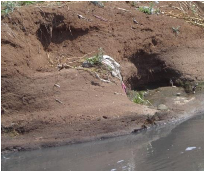
Figure 12. Pop out failure results to cavities. Source: Monene 2014: Photos taken on 17/12/2013 during wet season) and 5/9/2013 during dry season.
