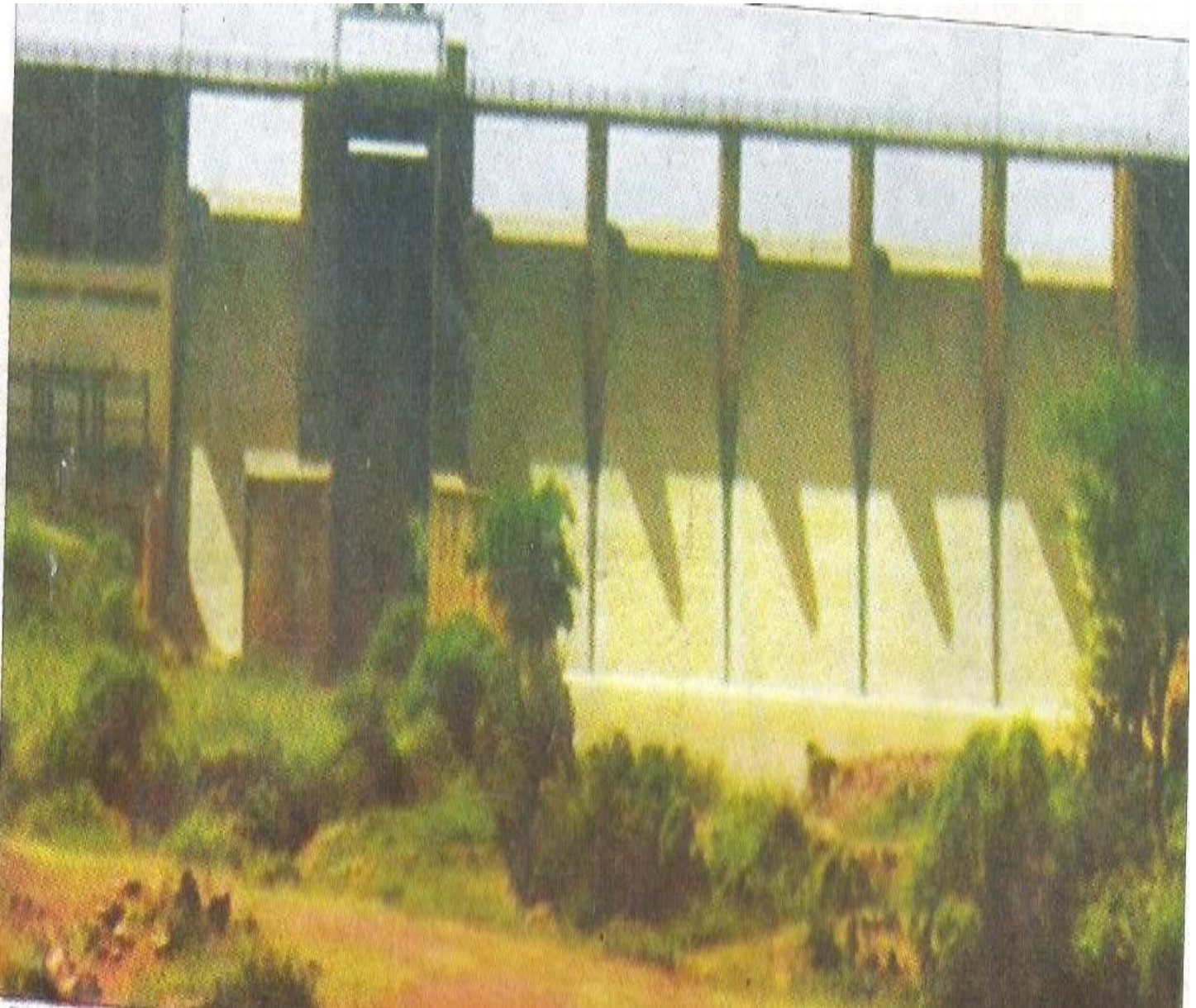
Figure 1. Dilapidated dam and abandoned farmland at Bakolori Irrigation site in Zamfara State.
