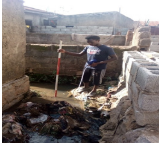
Figure 3. Constructed houses and domestic waste hindering flow of water.
